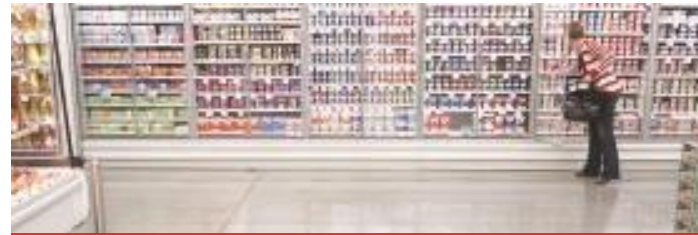
Refrigeration & Air Conditioning
